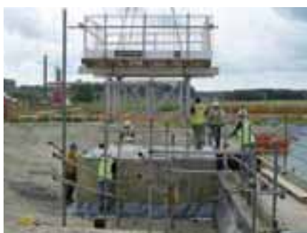
Ravenspurn Oil Platform The project comprises the construction of a 4m square 1.75m high concrete caisson in a dry dock...
