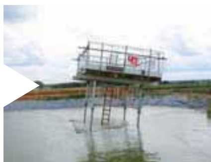
a platform is attached and the structure is floated into the lake...
